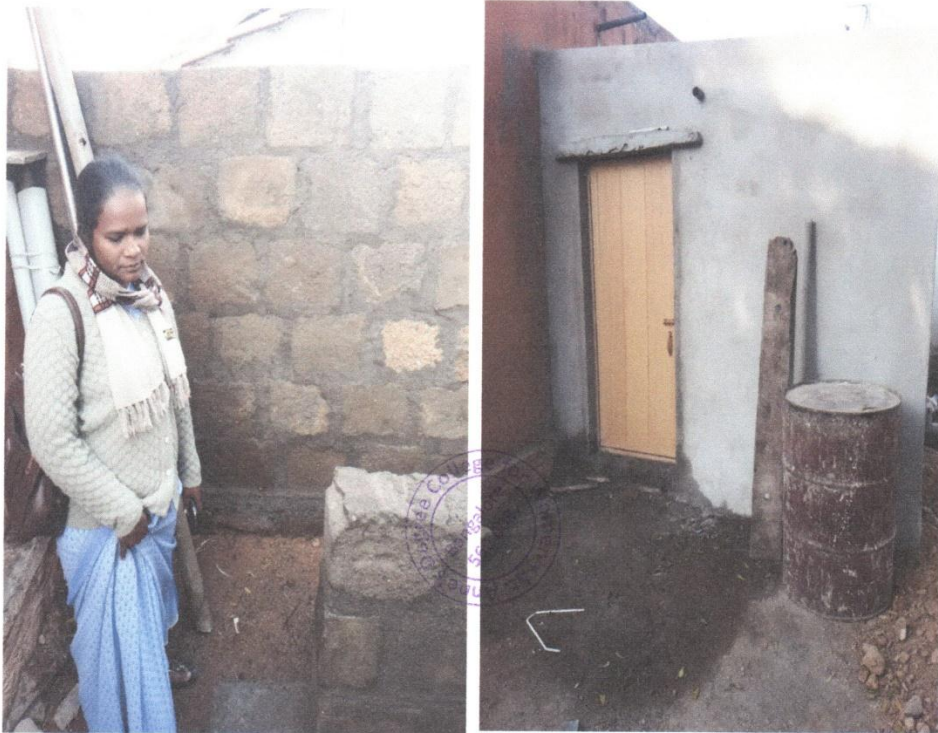
Photo No.02 INSPECTION BY Sr. Joshi (COLLEGE MANAGEMENT) CONSTRUCTION WORK IN PROGRESS
